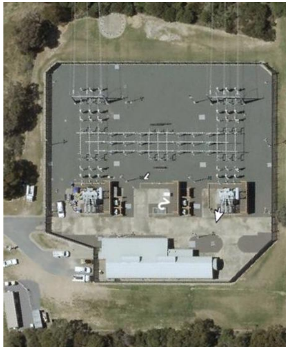
FIGURE 6: AERIAL VIEW OF GOLD CREEK ZONE SUBSTATION
