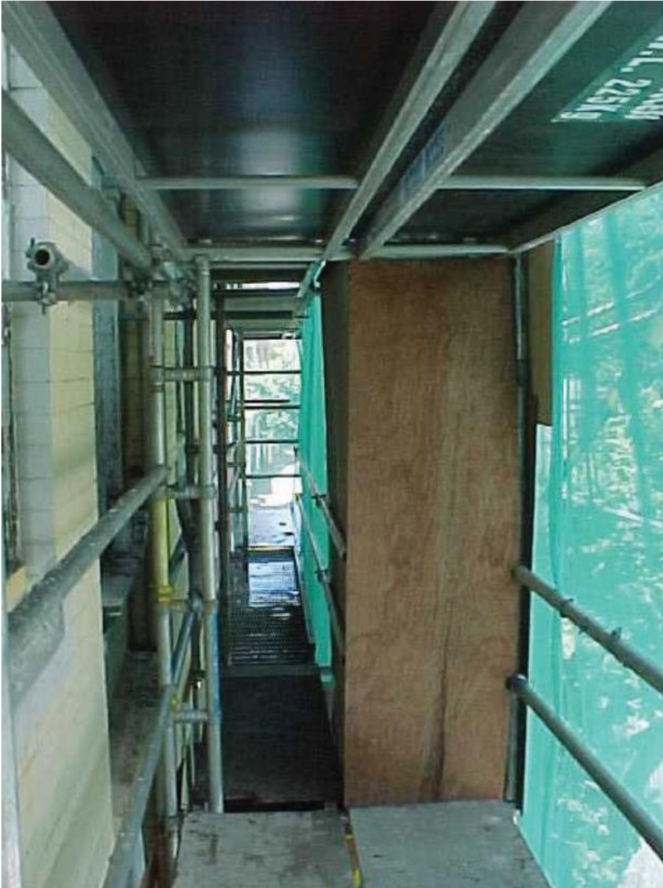
FIGURE 2. EXAMPLE OF HOARDING IN PLACE TO PROVIDE A BARRIER TO AN ENERGISED OVERHEAD LOW VOLTAGE NETWORK. SOURCE: SAFE WORK AUSTRALIA
