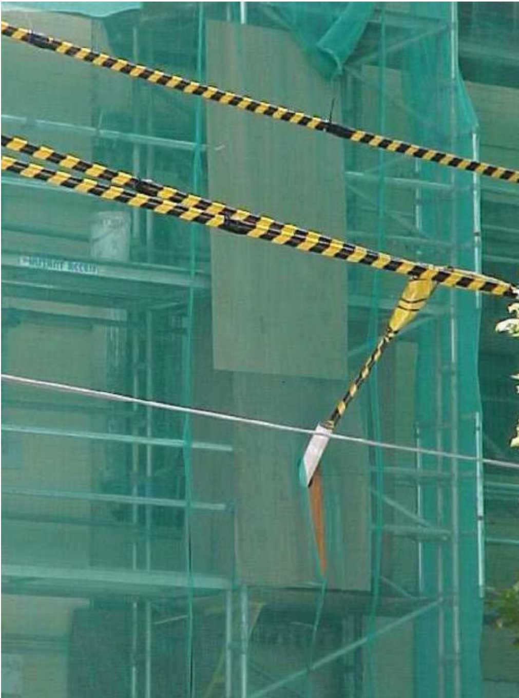
FIGURE 3. LOW VOLTAGE ELECTRICAL WIRES PASSING THROUGH A SCAFFOLD. APPROVED VISUAL INDICATORS, SUCH AS TIGER TAILS, RUN ALONG THE FULL LENGTH OF THE SCAFFOLDING PLUS A MINIMUM DISTANCE OF 5 METRES BEYOND EACH END OF THE SCAFFOLDING CAN HELP ISOLATE HAZARDS AND PREVENT DIRECT CONTACT OR “FLASHOVER” WITH ENERGISED OVERHEAD POWERLINES. SOURCE: SAFE WORK AUSTRALIA
